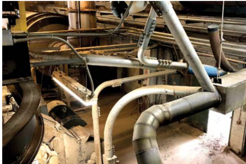
Installation of SonicAire dust control fans at Greene Team Pellet Fuel greatly reduced dust buildup on the rafters, improving the safety of the facility.
