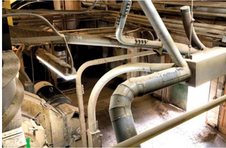
Before Greene Team Pellet Fuel installed SonicAire dust control fans, the plant's overhead rafters were laden with combustible dust, which posed a significant risk for a secondary explosion.
